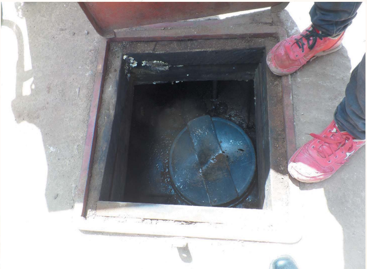
Figure 21: Plastic underground fuel storage tank found at one petrol station
