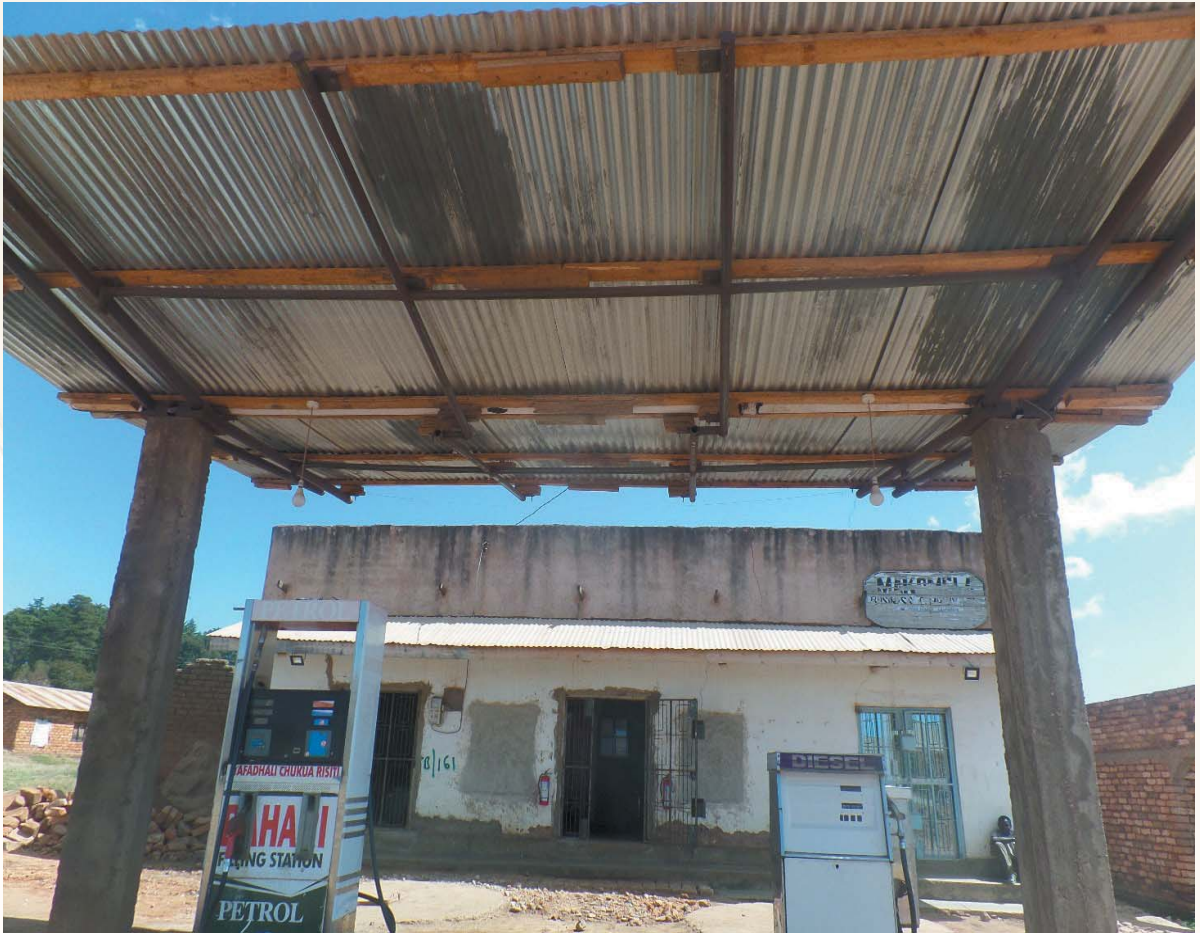
Figure 20: A petrol station canopy built of timber therefore posing HSE risks
